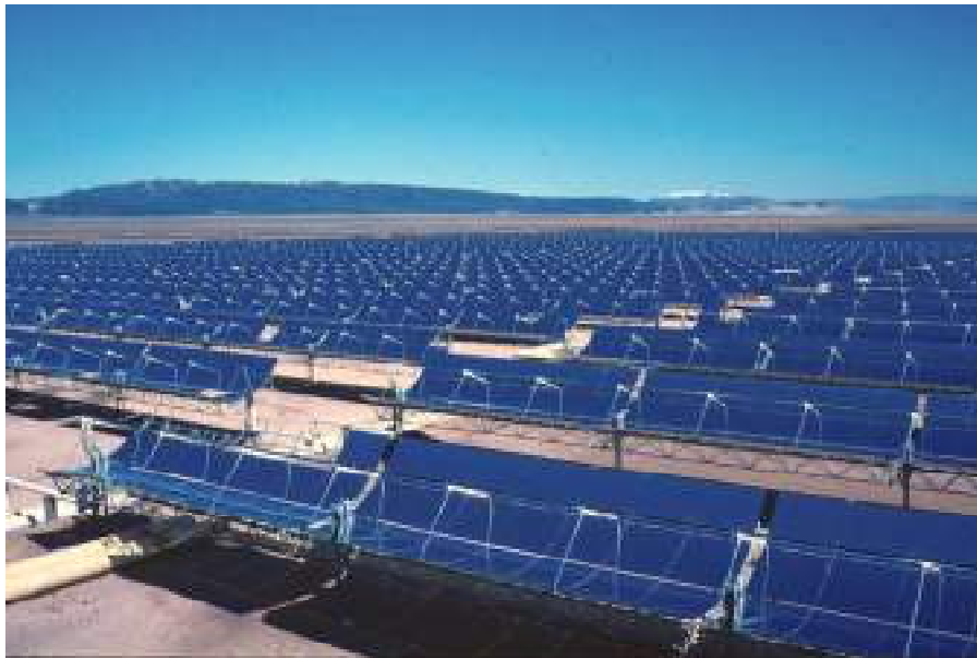
Figuur 18: CST-installatie in San Bernardino County, California. (Foto: Wikimedia Commons)
